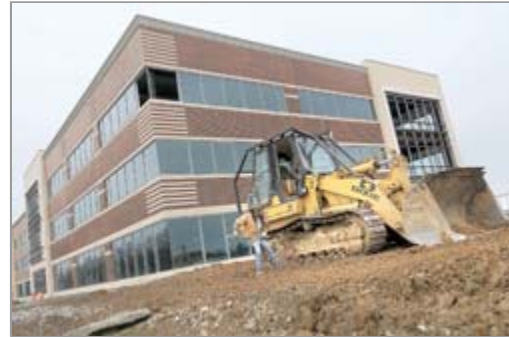
Construction is in progress at the North Gate Business Park in Harford County, at the north entrance to Aberdeen Proving Ground.
